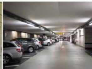
Parking lot lighting
