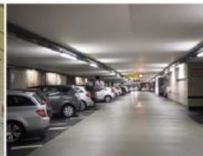
Parking lot lighting
