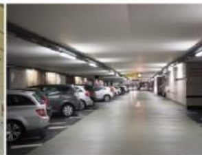
Parking lot lighting
