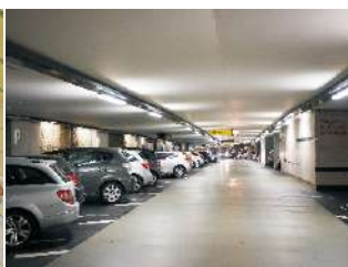
Parking lot lighting
