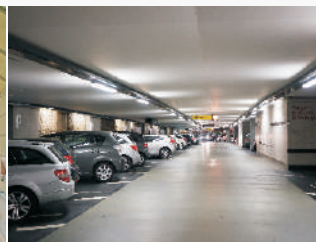
Parking lot lighting
