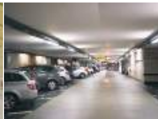
Parking lot lighting
